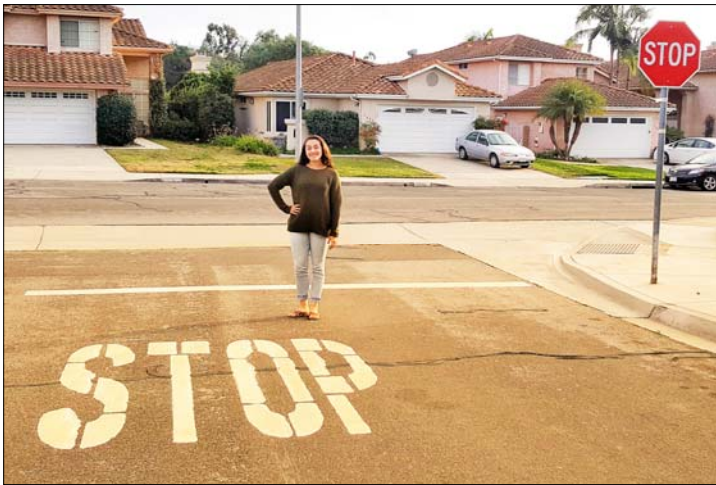
Madison Farfan with the repositioned stop sign , painted STOP on the street, and newly-installed ADA sidewalk ramps.
